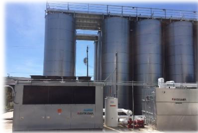
Ultra-low charge NH3 Chiller
