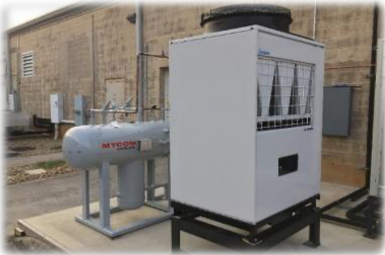
NH3 Chiller/ Pumped CO2
