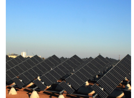
4 MW solar farm
