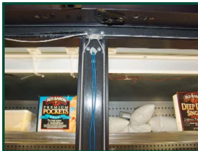
FIGURE 5. MULLION WITH DOORS AND MULLION ACCESS COVER REMOVED SHOWING WIRING FOR LIGHTS (BLUE) AND MULLION HEATER WIRE (WHITE)
