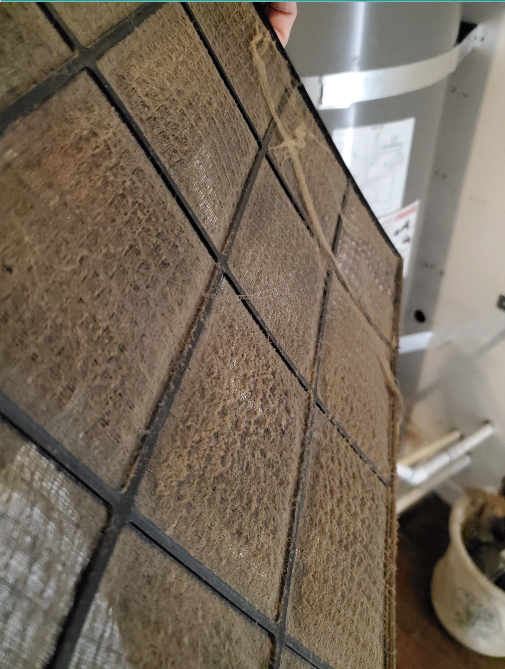
Filter cannot be removed for cleaning
