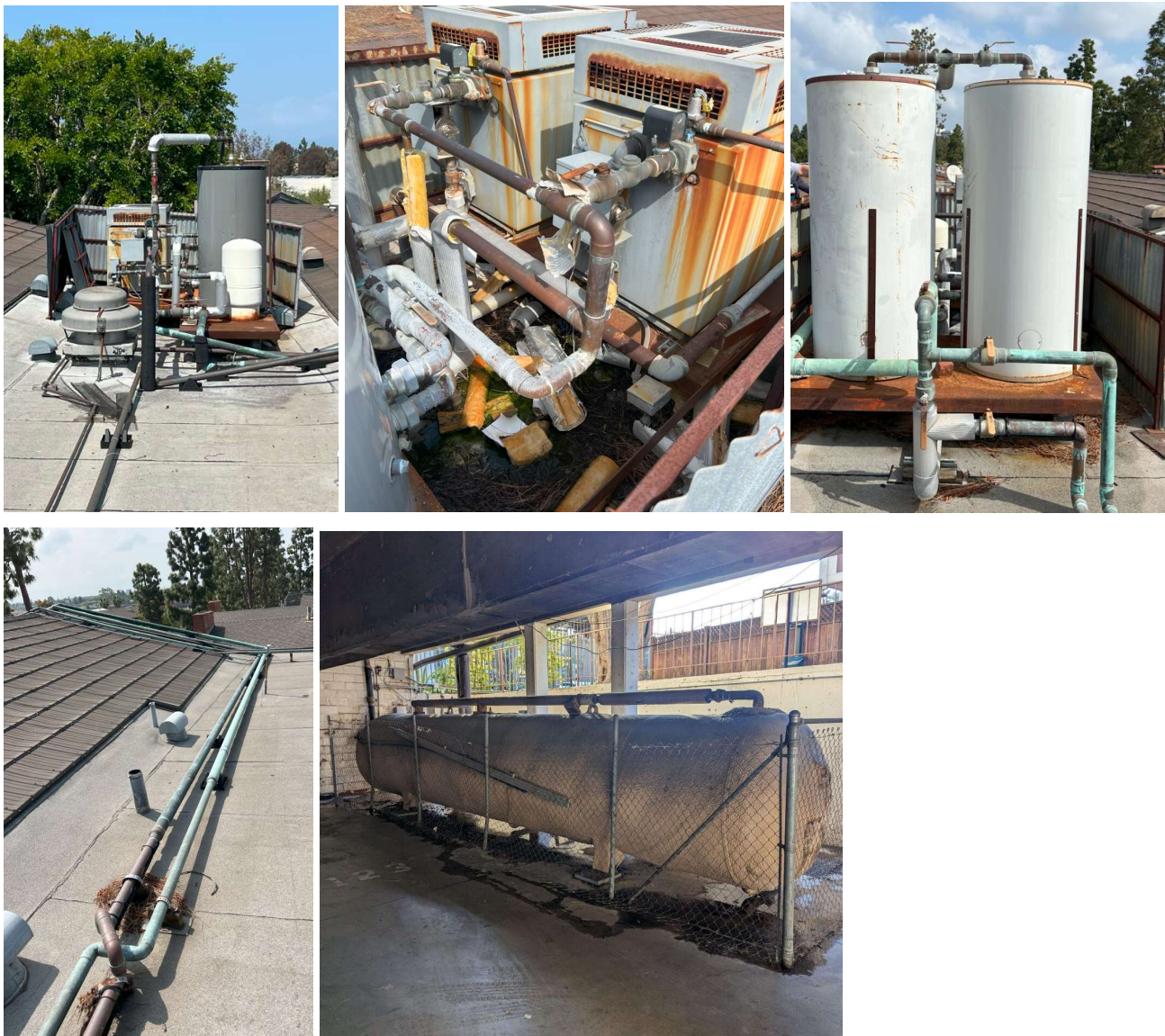
Figure 2: Existing Domestic Hot Water System
