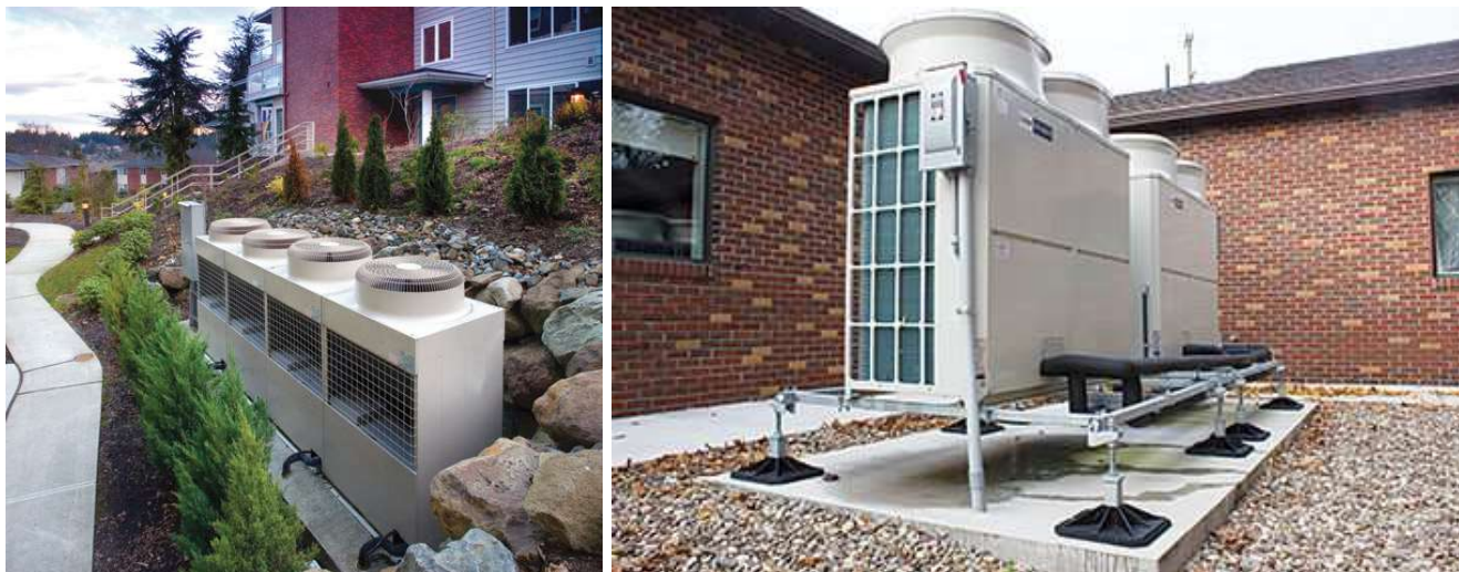
Figure 11: Central Heat Pump System Outdoor Units
