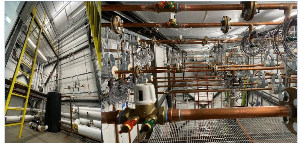
Hot Water Distribution System Testing
