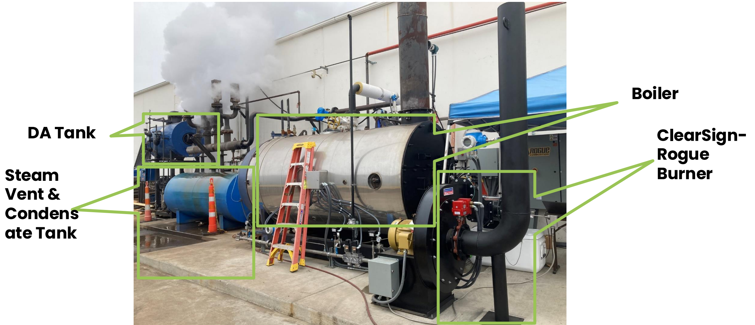
Figure 3. Boiler System Set-Up
