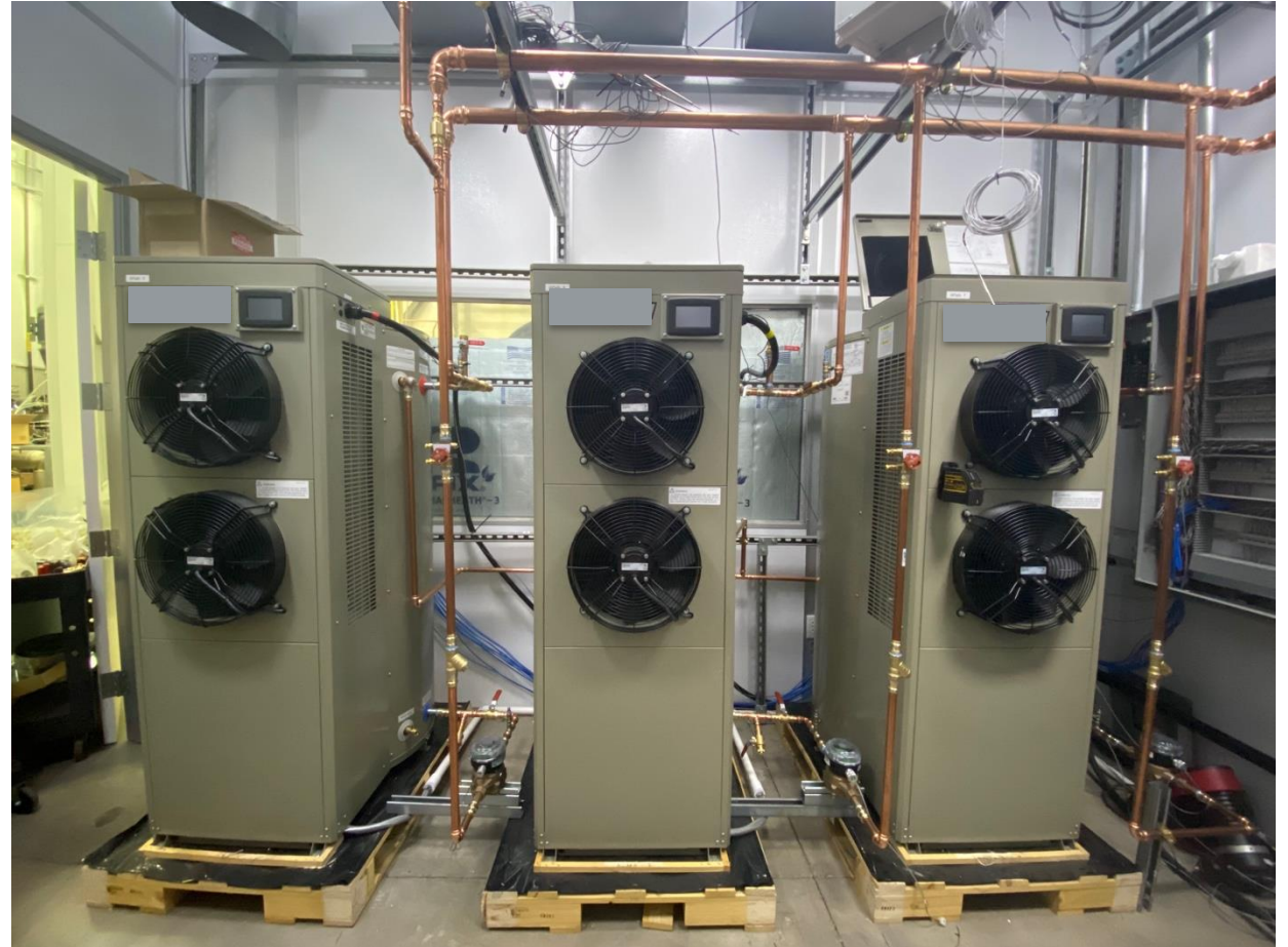
Primary heaters setup
