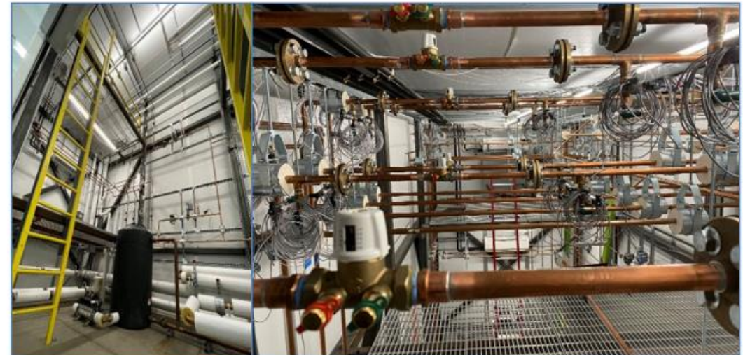
Hot Water Distribution System Testing
