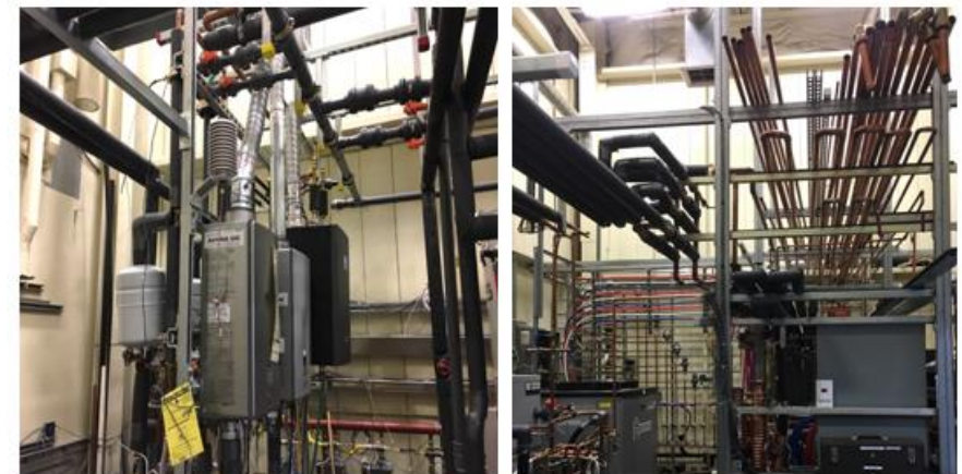
Commercial hot water system testing setup 2018
