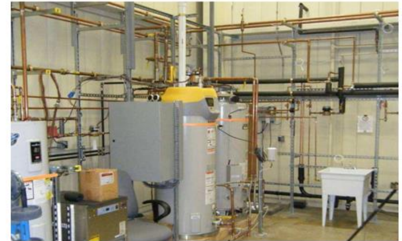
Commercial water heater system testing setup 2010
