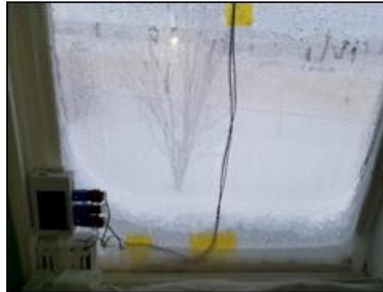
Condensation and ice buildup on existing double-pane
