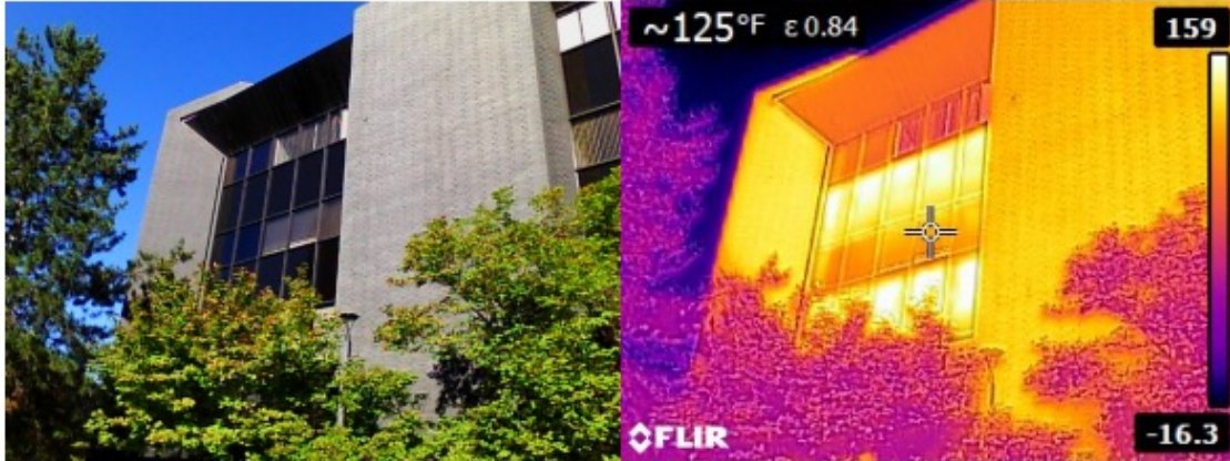
FIGURE 4 – THERMAL IMAGE OF PRE-INSTALL SE (SUNNY SIDE) GLAZING EXTERIOR (9/2/20 8AM – OAT=63 °F)
