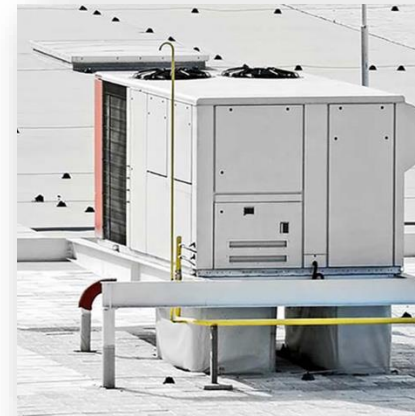
Efficient Rooftop Units
