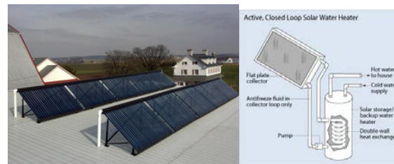
FIGURE 28. EVACUATED TUBE SOLAR WATER HEATERS 55
