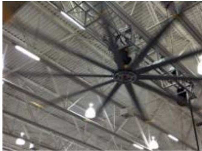
FIGURE 7. HIGH VOLUME LOW SPEED FANS (PHOTO TAKEN AT WORLD DAIRY EXPOSITION 2012)
