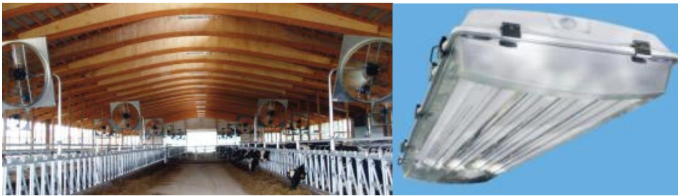
FIGURE 23. HIGH INTENSITY FLUORESCENT LIGHTS
