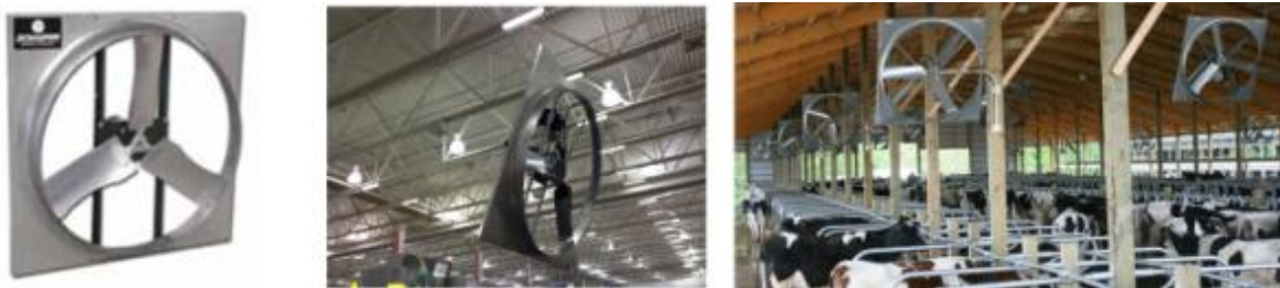
FIGURE 9. PANEL FANS (PHOTO COURTESY: GEA FARM TECHNOLOGIES)
