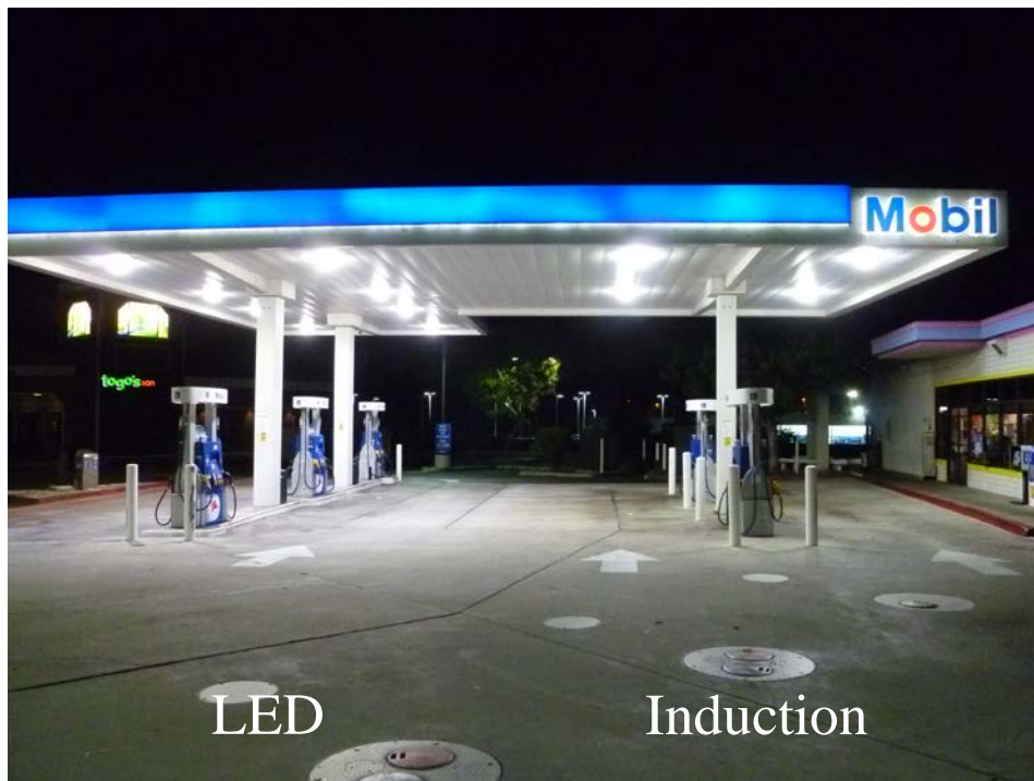
Figure 5: Side-by-side comparison of LED retrofit (left) and Induction retrofit (right).
