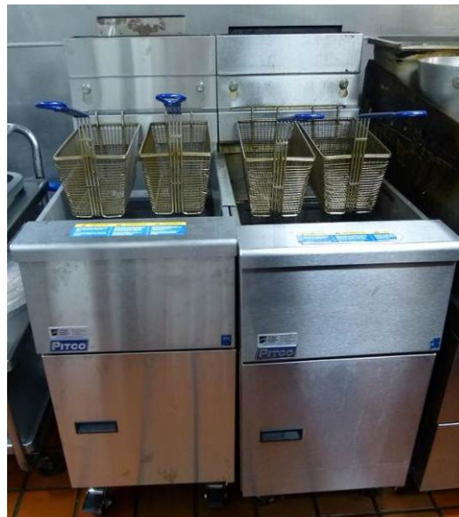
FIGURE 27. TRUEBURGER FRYERS: FRY BANK WITH REPLACEMENT FRYER (LEFT SIDE)
