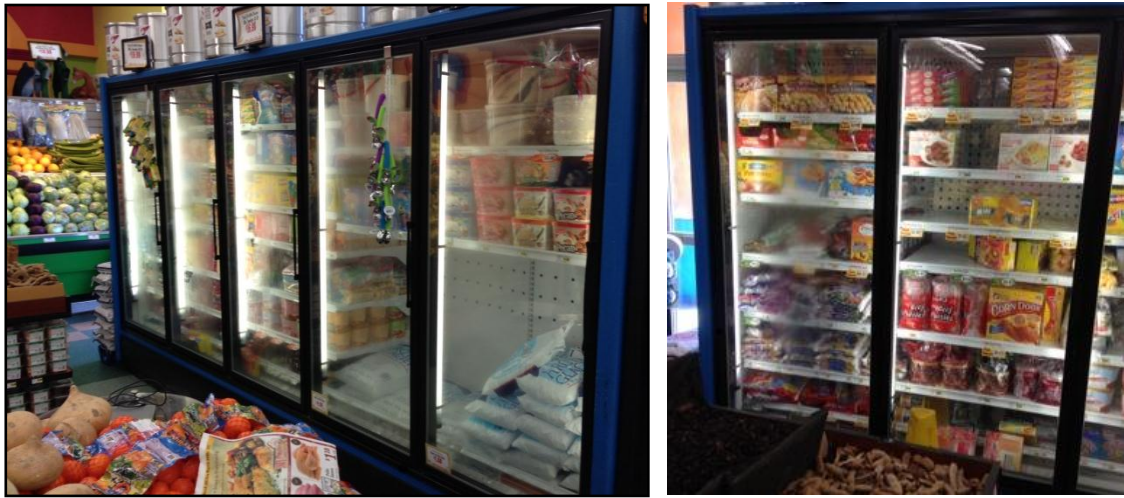
FIGURE 3: DOORS WITH CONDENSATION
