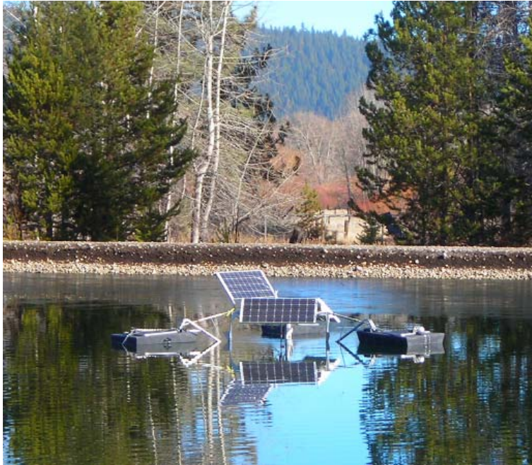
Figure 1 An Operating SolarBee Unit
