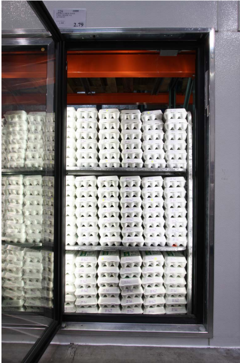
Figure 4.4: Test-case LED Lighting System
