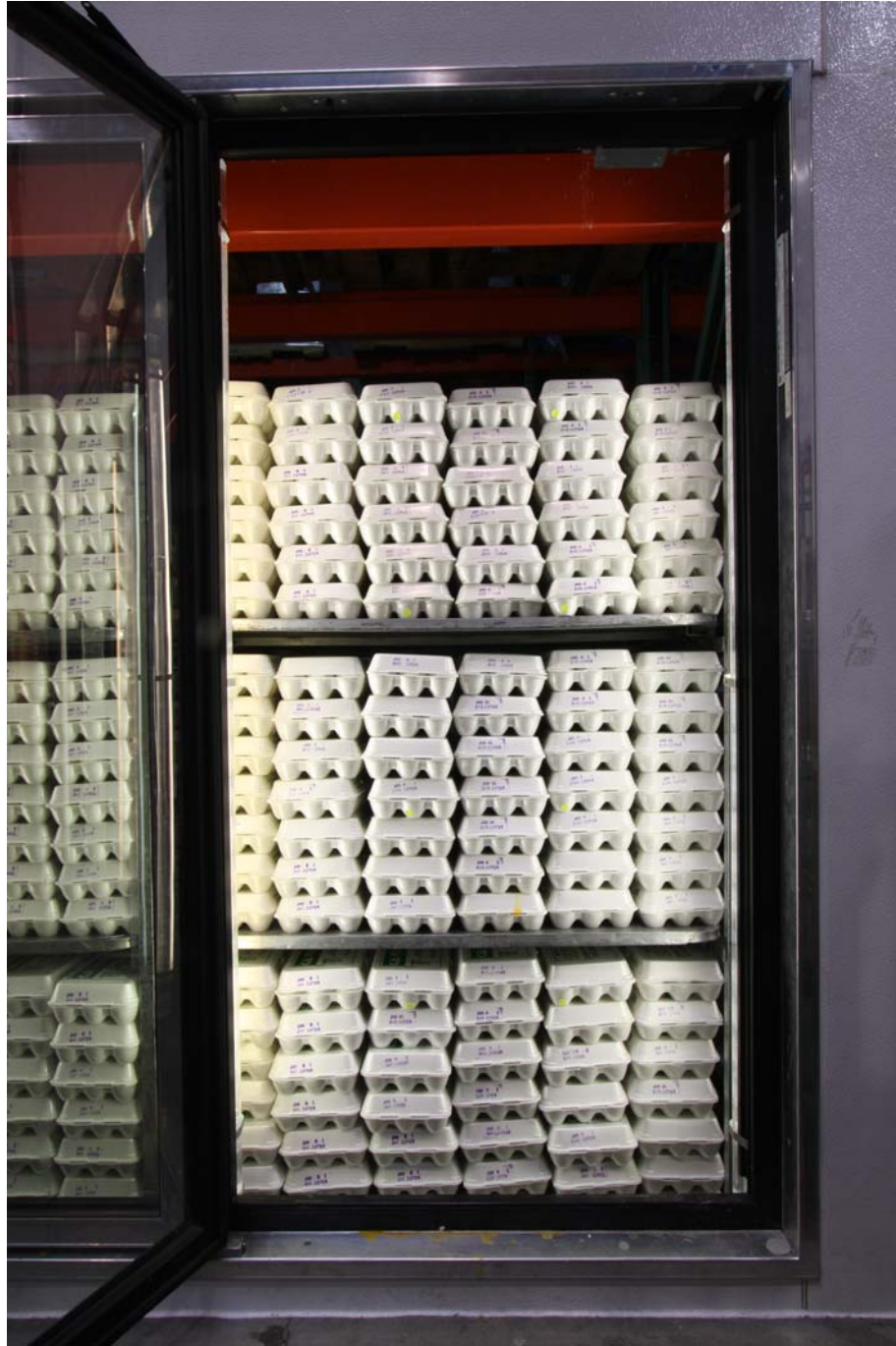
Figure 4.3: Baseline Fluorescent Lighting System
