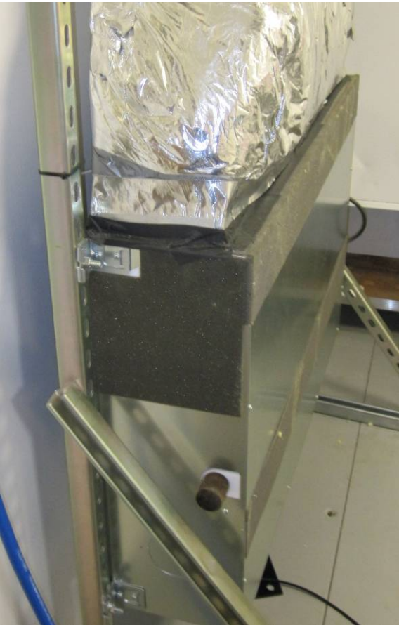
Indoor Air Handler
